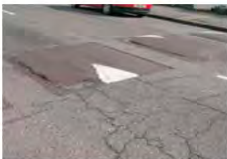
Potholes and differently coloured Surface may cause a loss of grip. (source: Craig Carey-Clinch, MCI, UK)
