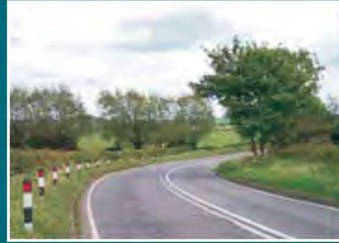
This bend has been fitted with marked posts to make it more predictable (source: A.J.Sharp IHIE)
